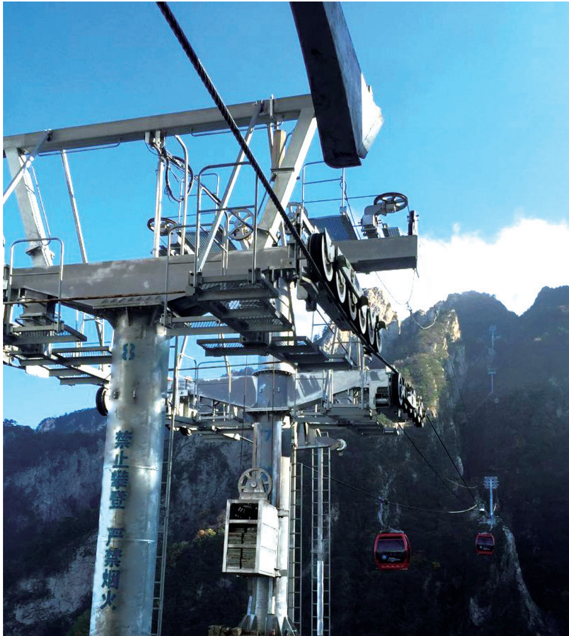
GOLDEN PEAK, LAOJUN MOUNT, 8-MGD LUANCHUAN COUNTY, HENAN PROVINCE 河南栾川老君山金顶脱挂索道
